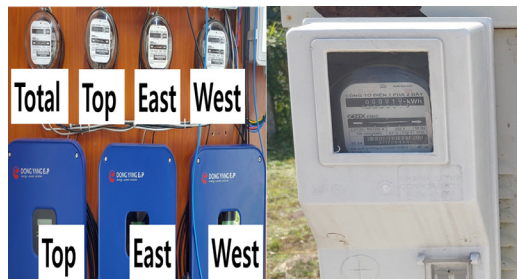
Fig. 6. The power meter connected to each solar inverter and the main distribution board power meter
